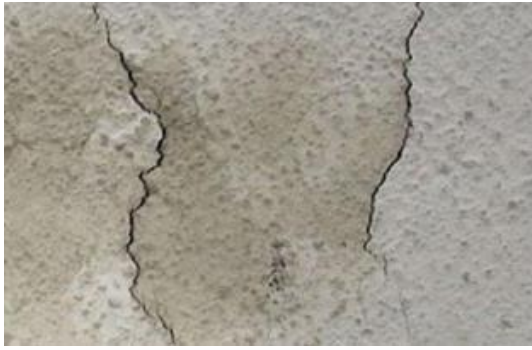
Figure 2.3 Early drying shrinkage on a slab roof. a
