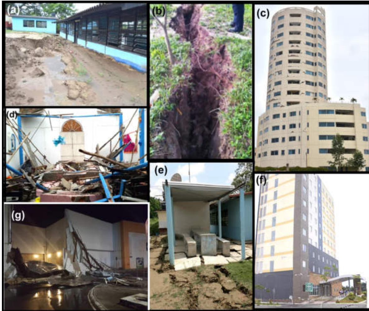
Figure 5.2. Evidence of major damage caused in Centro, by September 8, 2017, M_w 8.2 earthquake. (a) and (b) failure of sediments, landslides and liquefaction process, (c) shows the structural damage observed in the Zafiro Tower a building 16 stories high, (d) the roof of the catholic church de Nuestra Madre de Asunción de María, (e) failure of sediments and liquefaction process in a elementary school, (f) The Hotel Fairfield Marriot tower damaged during the event, and (g) the roofing of the Sendero mall collapsed.
